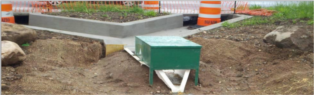
H-Flume: Example of the h-flume that will be used at the inlets. Flumes used at GIG will likely not have the green box as shown above.
