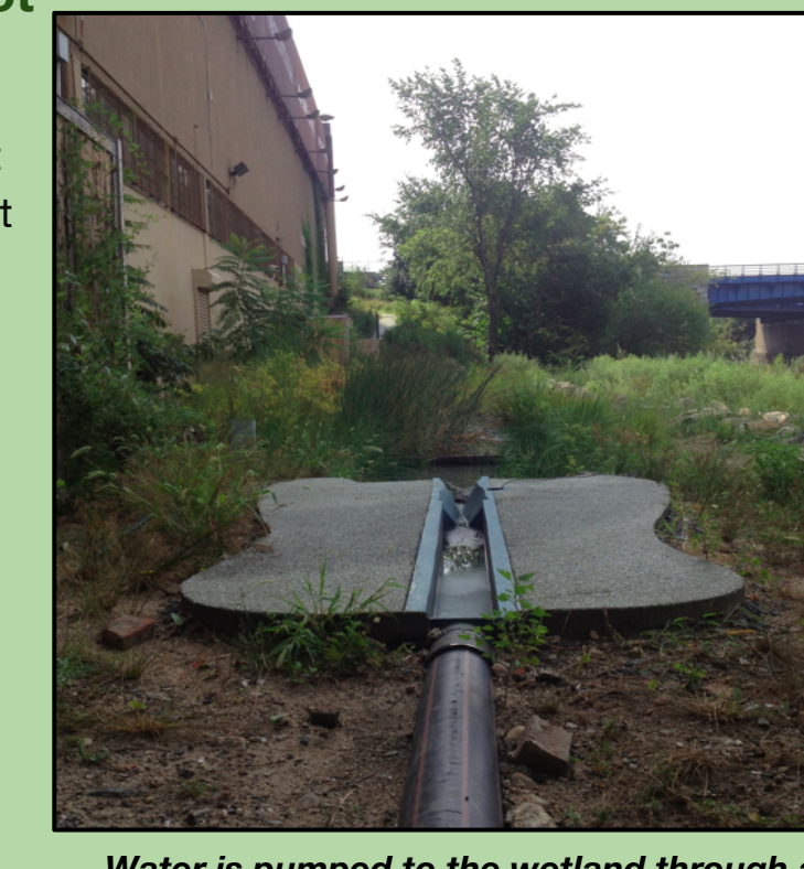
Water is pumped to the wetland through a trapezoidal flume to measure inflow.
